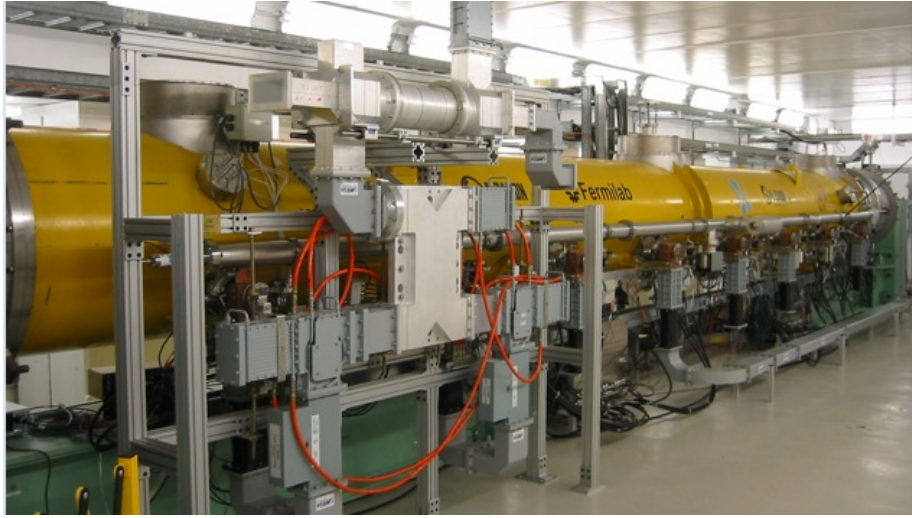
Figure 12. The first 1.3 GHz SRF cryomodule installed in the FAST/IOTA facility.
