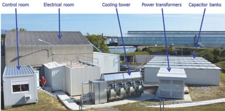
Fig. 3.18. The new power system for the PS main magnet.
