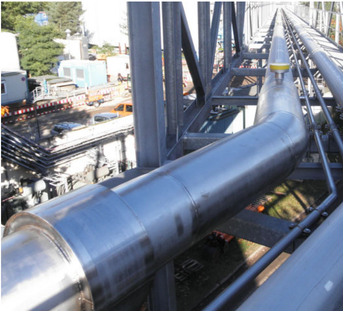
Fig. 9.29 The XFEL/AMTF cryogenic transfer line installed on the pipe bridge ( courtesy Kriosystem Ltd.)
