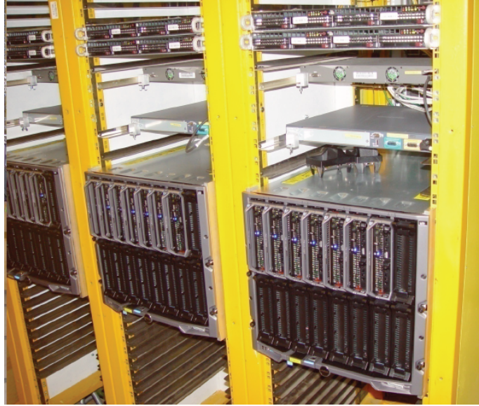
Figure 4.10: View of a section of the LHCb Event Filter Farm, where the software trigger is executed.
