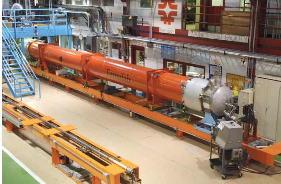
Figure 0.1: LHC quadrupole production magnet installed at the Magnet Test Facility.
